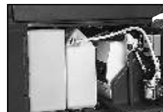
Tanks and Hot Water Heater
